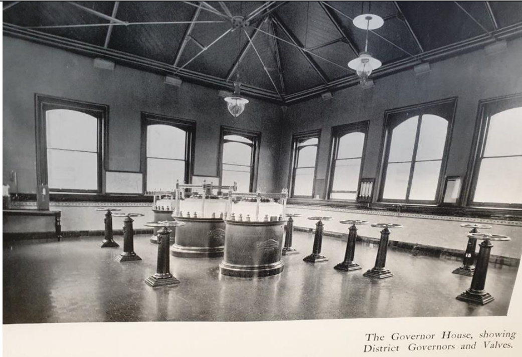
Fig. 5: Inside the Governor House showing district governors and valves. From Reading Gas Company: A Retrospective - Douglas H Helps (1912)
